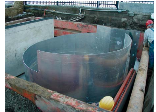
Stormwater treatment system
