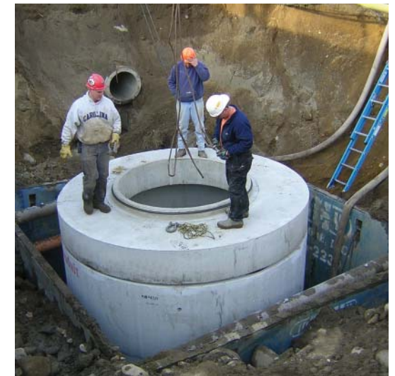
Stormwater treatment installation, Lake George
