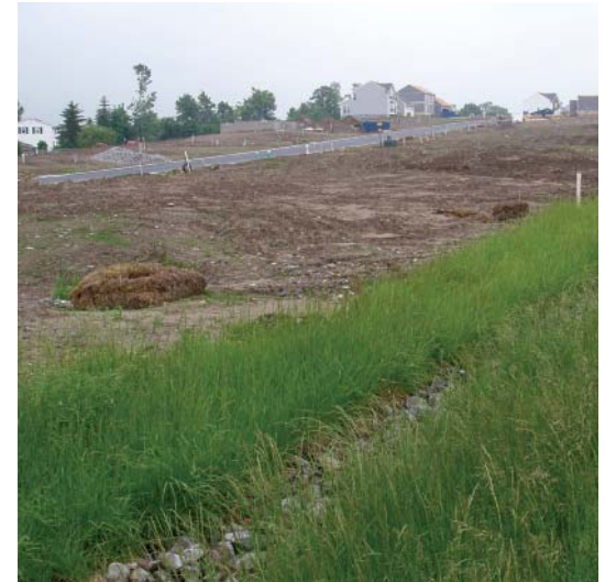
Construction site erosion
