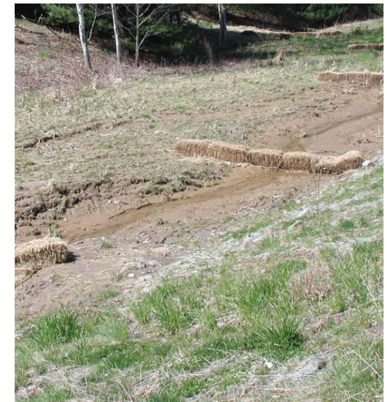
Improper use of control measures
